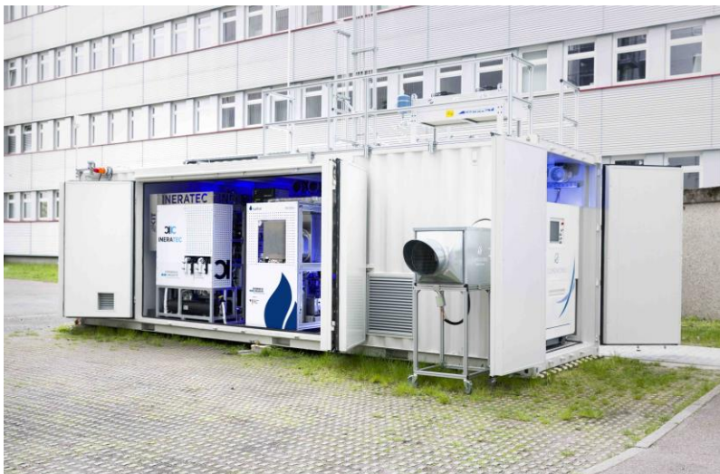
The world's first integrated Power-to-Liquid (PtL) test facility to synthesize fuels from the air-captured carbon dioxide. (Photo: P2X project/Patrick Langer, KIT)
