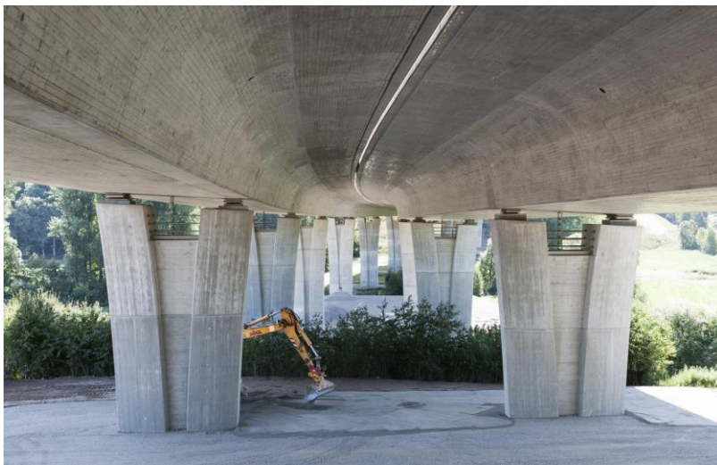
KIT researchers develop a process to detect damage of bridges at an earlier point of time. (Photo: Markus Breig, KIT)
