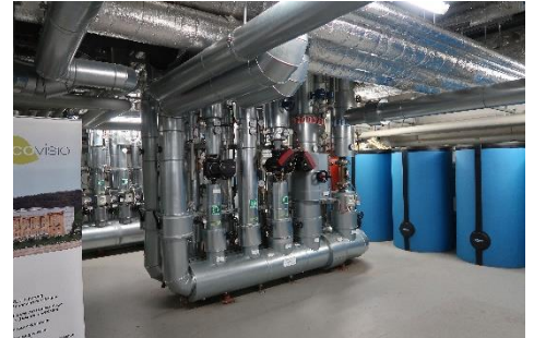
The aquifer storage system in Bonn supplies up to 80% of the heat and cold in three buildings covering a total area of 60,000 m 2 . (Photo: Paul Fleuchaus, KIT)
