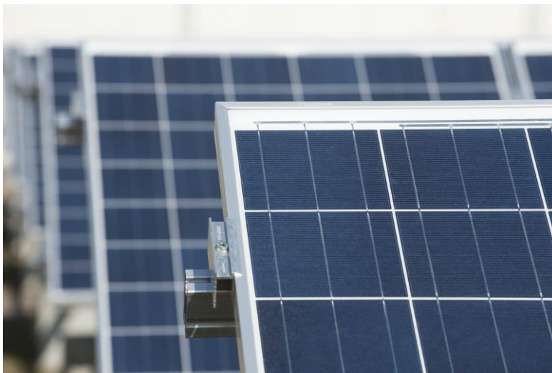
The solar park on Campus North of KIT generates sustainable energy to operate some of the large-scale research facilities. (Photo: Martin Lober/KIT)
