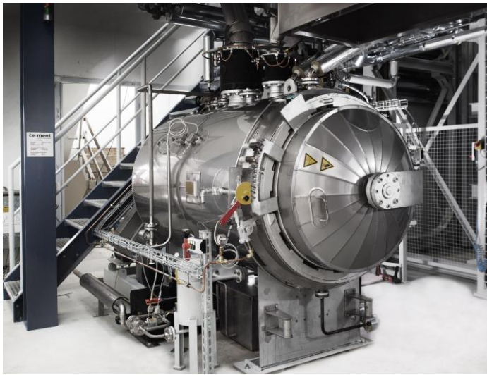
This is where the innovative cement is produced: The Celitement pilot plant on Campus North of KIT. (Photo: Markus Breig)
