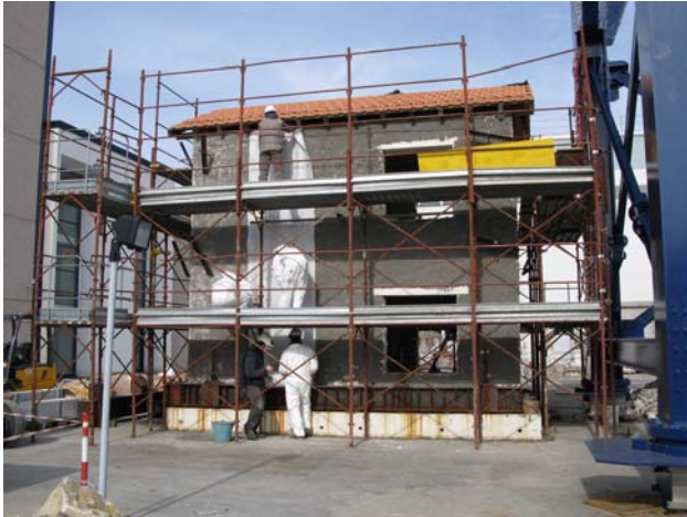
Large-scale test in Pavia: A greatly damaged building is reinforced with seismic wallpaper and then tested on a vibrating table. (Photo: Moritz Urban)
