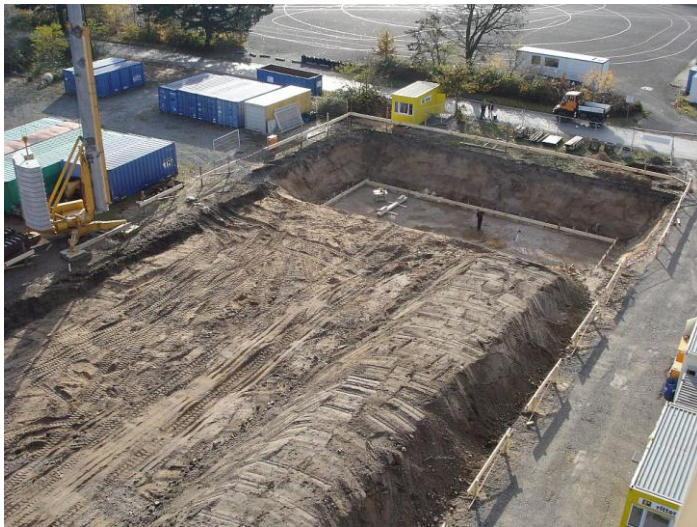
Start of construction on the site of the Mackensen barracks: Excavation of an area of about 1500 square meters. (Photo by: Thorsten Dreher)
