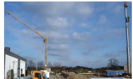
Construction site on the premises of the Mackensen barracks. (Photo by: Michael Frey)
