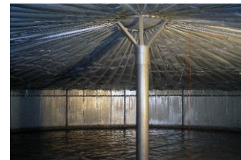
Interior of the test tank. The gas membrane partly lies on the support construction. (Photo: Rosemarie Wagner, KIT)
