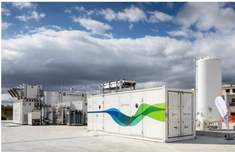
The demonstration plant at Troia, Italy, combines a new type of microreactor for methanation with an innovative liquefaction plant. The CO 2 needed is extracted from ambient air. (Photo: Domenico Grossi)
