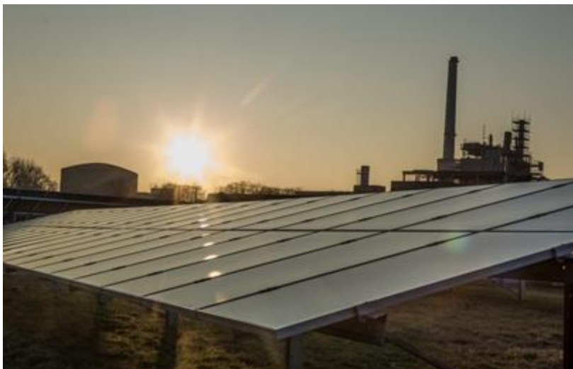
Sustainable technologies, such as solar power generation at KIT, are of crucial importance to the transformation of the energy system. (Photo: KIT)
