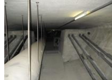
The tensioning ropes to be checked are located in the hollow concrete box of the bridge. (Photo: S. Siegel/KIT)
