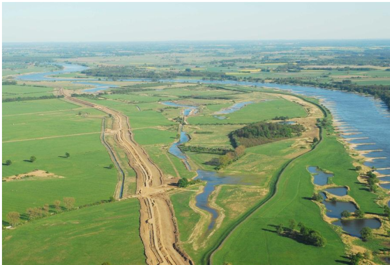
Rerouting of levee: The river Elbe and the old levee are visible on the right, the new levee on the left. (Aerial photograph: Jochen Purps)
