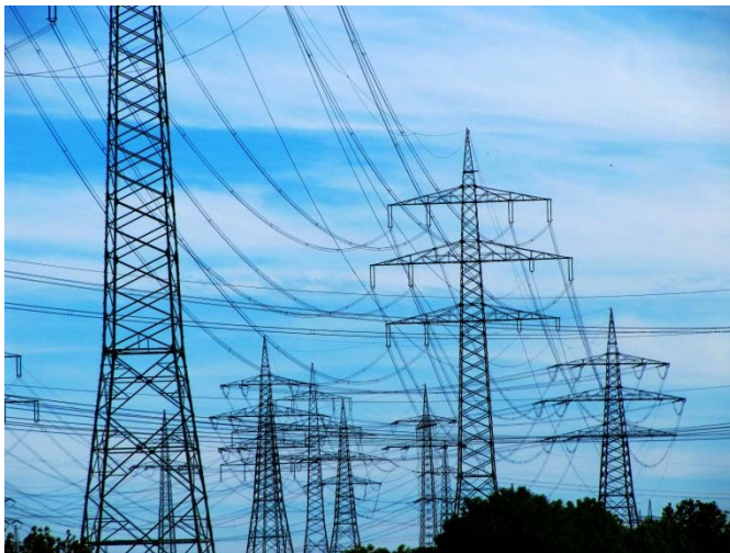
Electricity grids: The energy turnaround requires new technologies for a reliable supply. (Photo: Rainer Sturm/pixelio.de)
