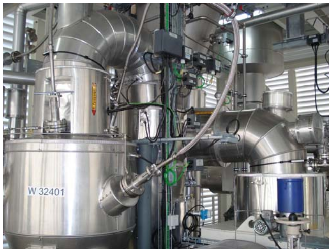
Production of bioliqSynCrude® on KIT Campus North: The plant will now be extended by the two remaining stages for the production of synthesis fuel. (Photo: KIT)
