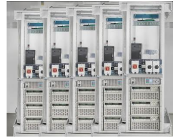
The “SafetyFirst” project studies safety, quality, and grid suitability of home storage systems for power produced by photovoltaics systems at more than 20 test rigs. (Photo montage: KIT)
