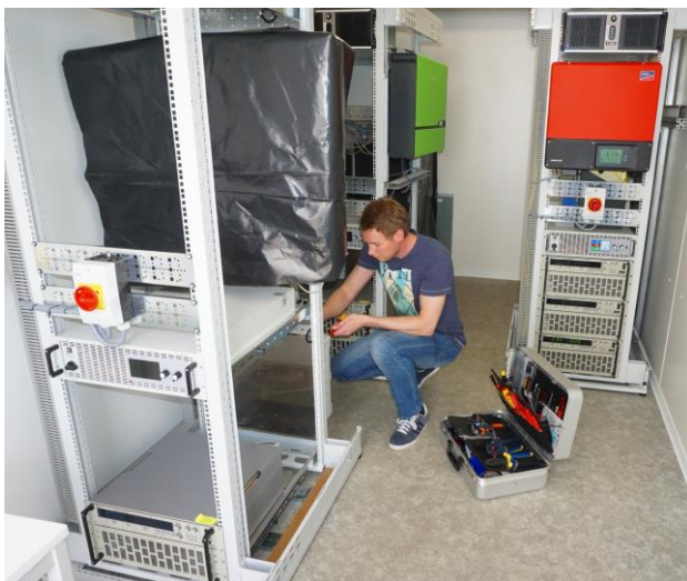
KIT's test rigs to analyze safety, quality, and grid suitability of home storage systems for electricity generated by photovoltaics systems. (Photo: KIT)
